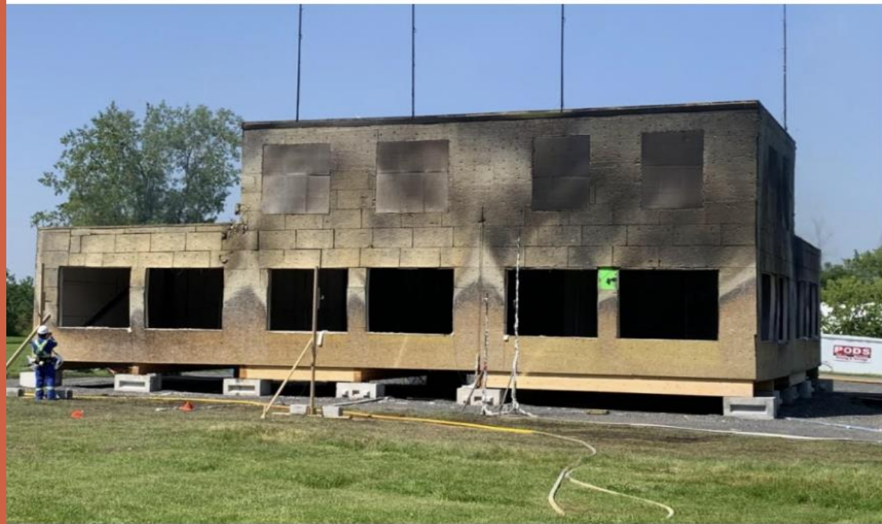
State of mass timber structure after fire research test.
