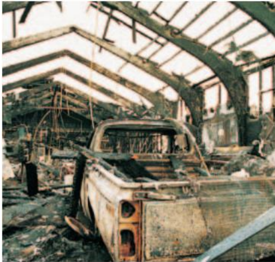
Aftermath of the fire at Turbotech, Inc. in Vancouver, WA. Glulam remained standing while the rest of the so-called “fireproof” building collapsed.
