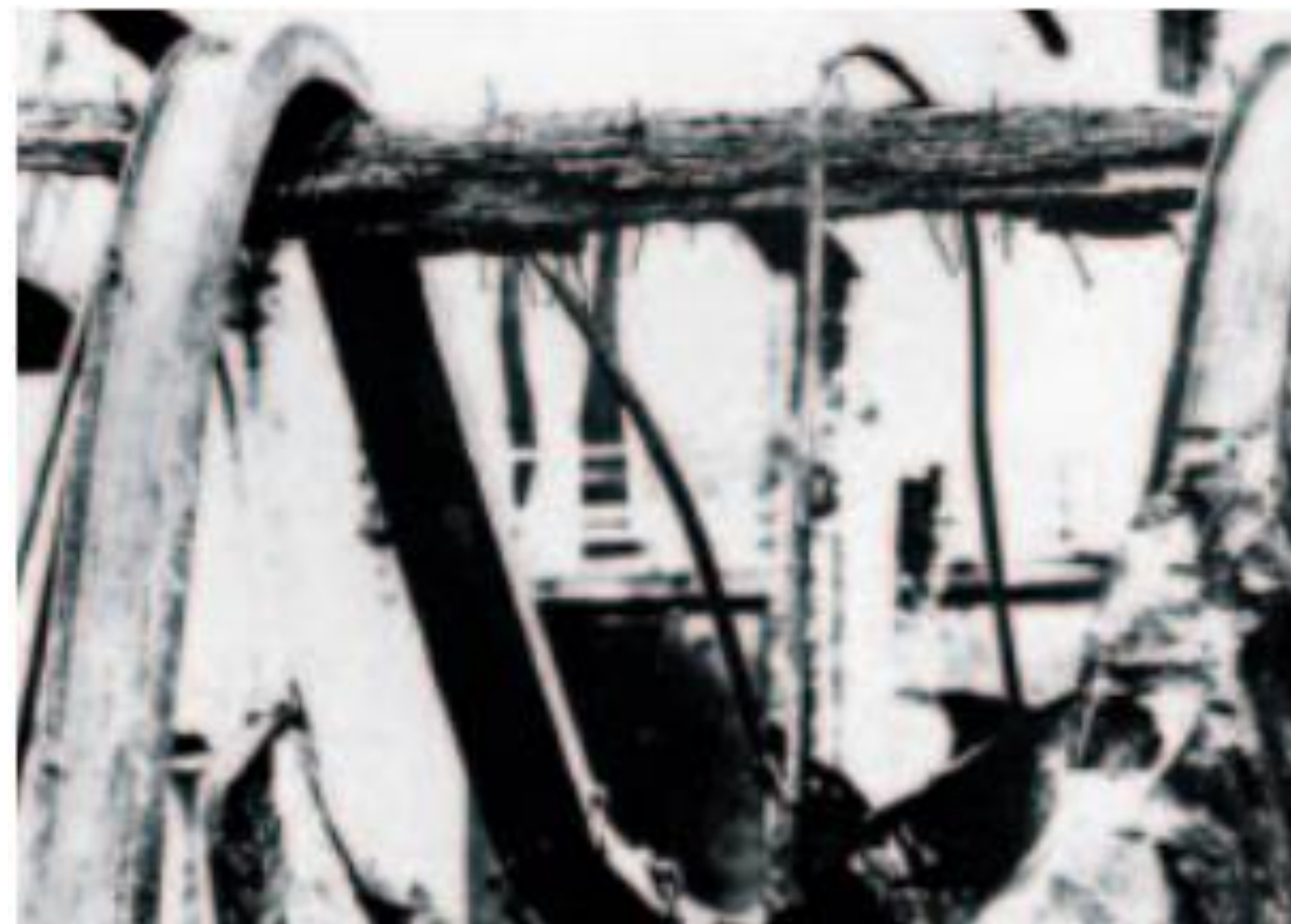
Steel beams have melted and collapsed over charred timber beam which, despite heavy damage, remains in place.
